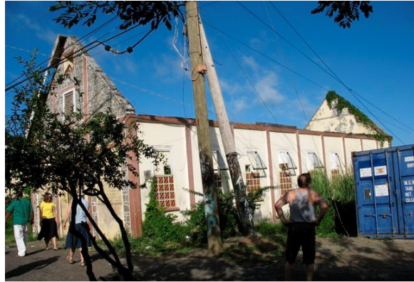
One of many damaged churches visited.
